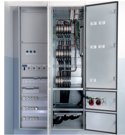
Each enclosure and cell centre can be dimensioned carefully for their intended purpose.
